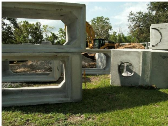
HunterPark a couple of months ago with the drain pipes which were put down the middle of the park.
